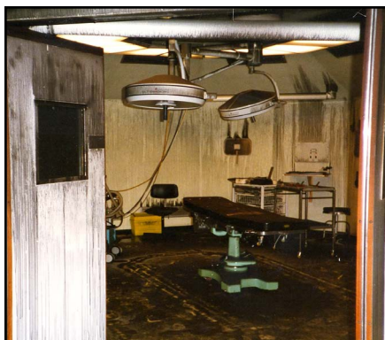
The operating theatre damaged after a cigarette was discarded in a waste paper basket
